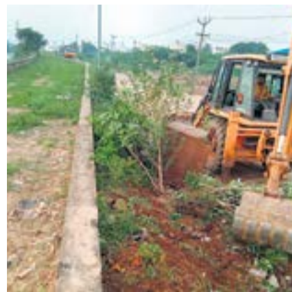
Work is in full swing for the rejuvenation of the Ayanambakkam Lake. The project is likely to be completed before Dec, 2025
